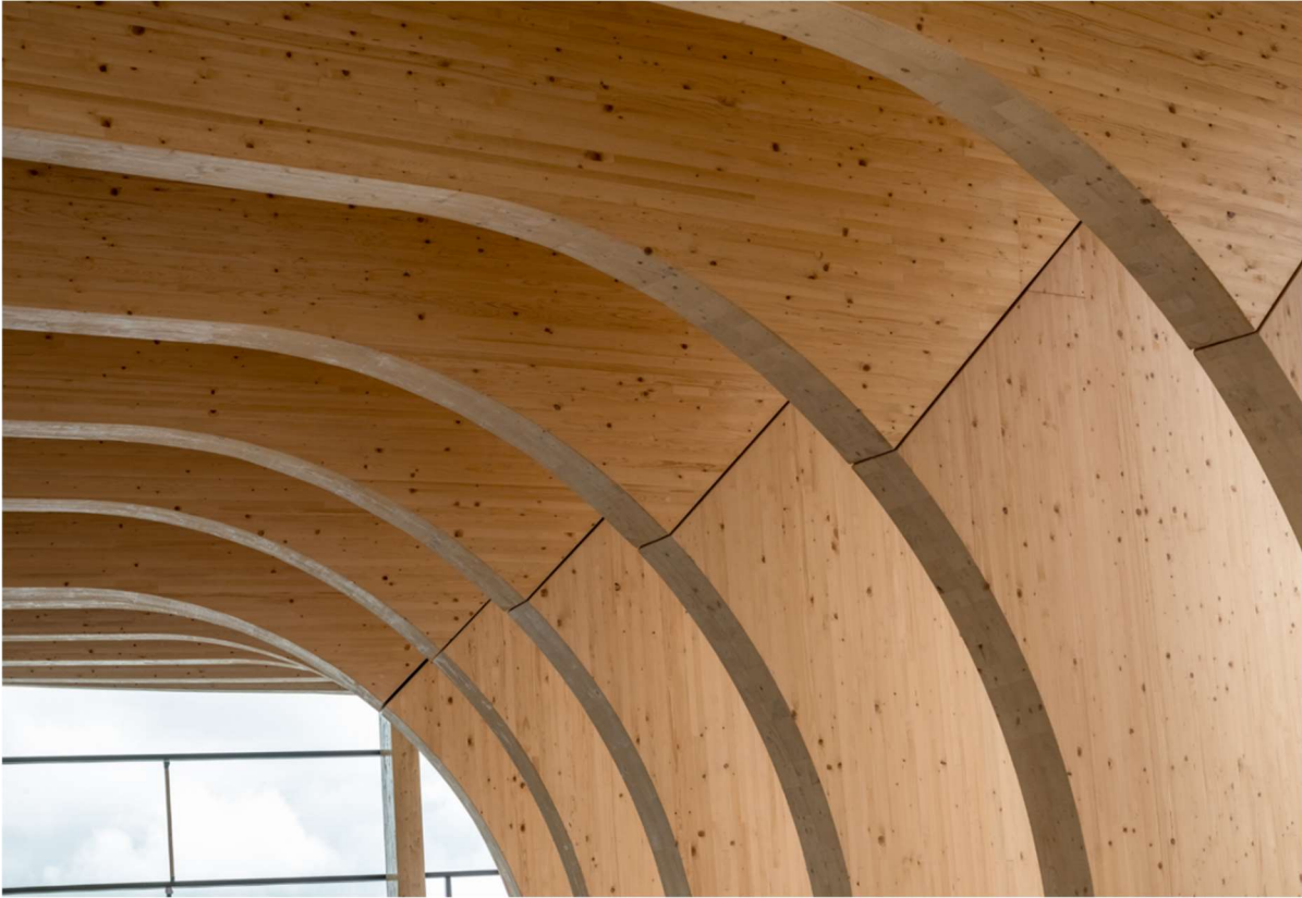
Picture 9: Tree trunk corner as signature detail, all steel connectors are embedded
