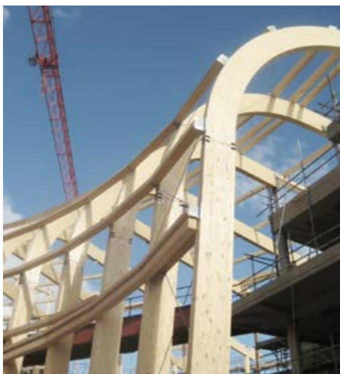
University of Reading, arched façade supports General butt joint on building site
