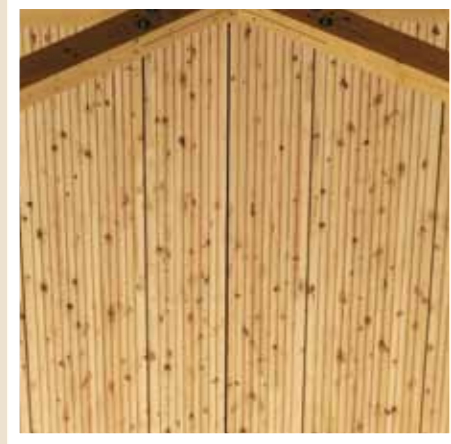
Production Hall for "Weißhaidinger Engineered Timber": WIEHAG Freespan girders combined with WIEHAG Profidec roof elements made of pine and an acoustic surface
